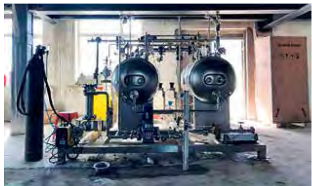
Homemade sewage treatment systems
